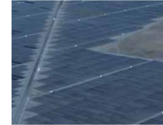
GES 4-Bor-3 SPP (Installed Capacity MWp 130)
